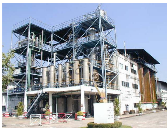
Fig. 6.5.2. Ethanol production plant in Thailand.
